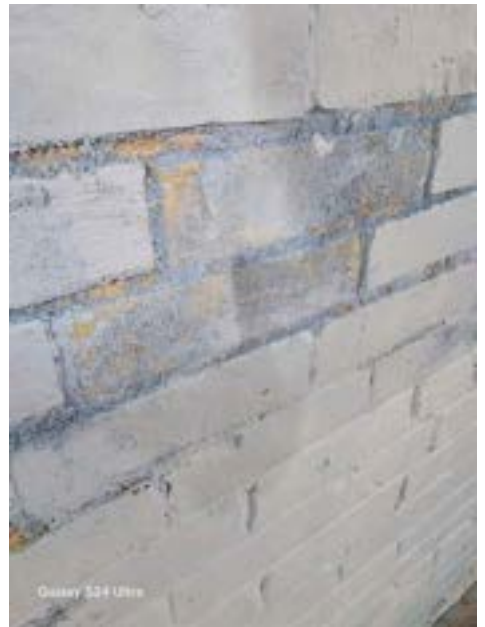
Foundation Photos/ old moisture stains
