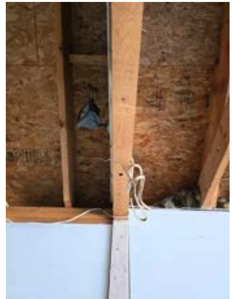
Light in garage is disconnected
