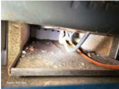
Debris observed in burner cabinet. Recommend clean/tune by qualified HVAC technician
